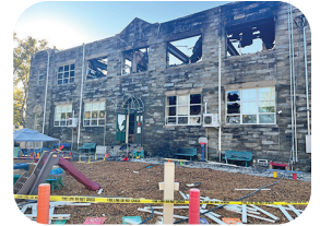
An October fire gutted one of the two school buildings at St. Francis of Assisi. Photo by Terrence Casey
